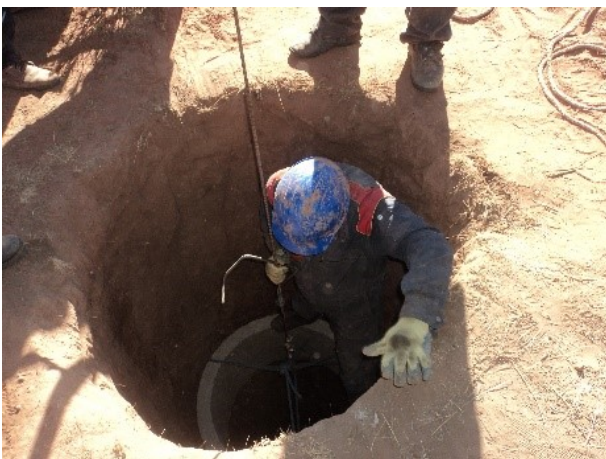
One of the wells at Chullunkani being installed, ring by concrete ring.
